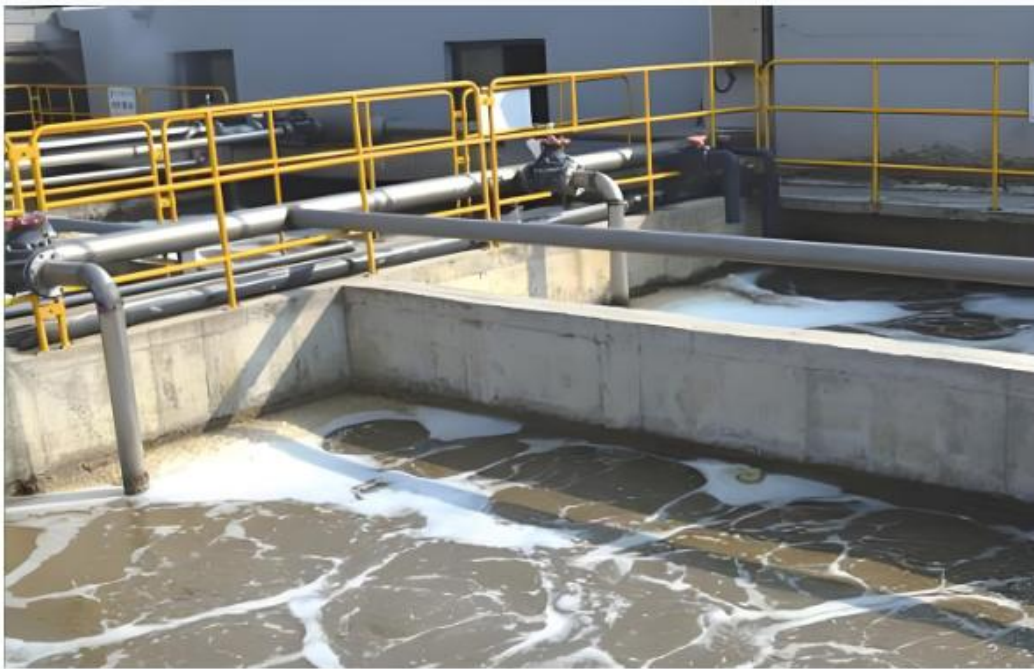
Galvanized Steel Drain Pipe
